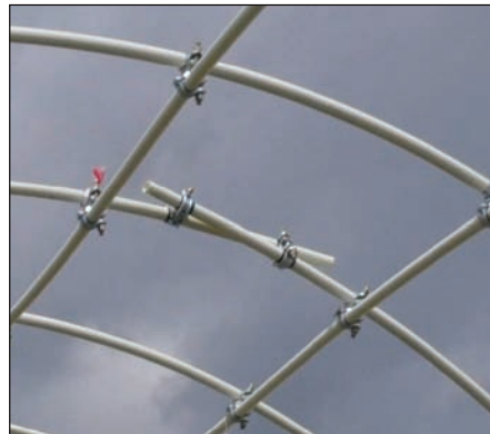
Fig. 21: Poor connection between two beams
