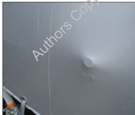
Fig. 22: Connection bolt that can damage the canvas
