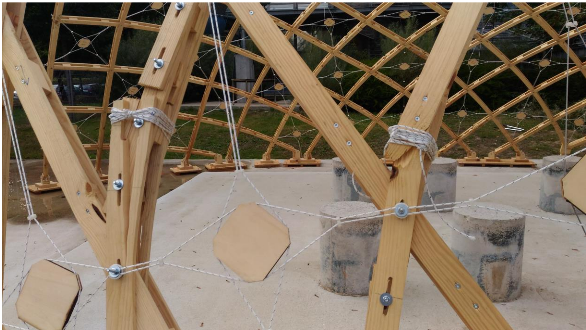
Figure 6 Failure of longitudinal joints
