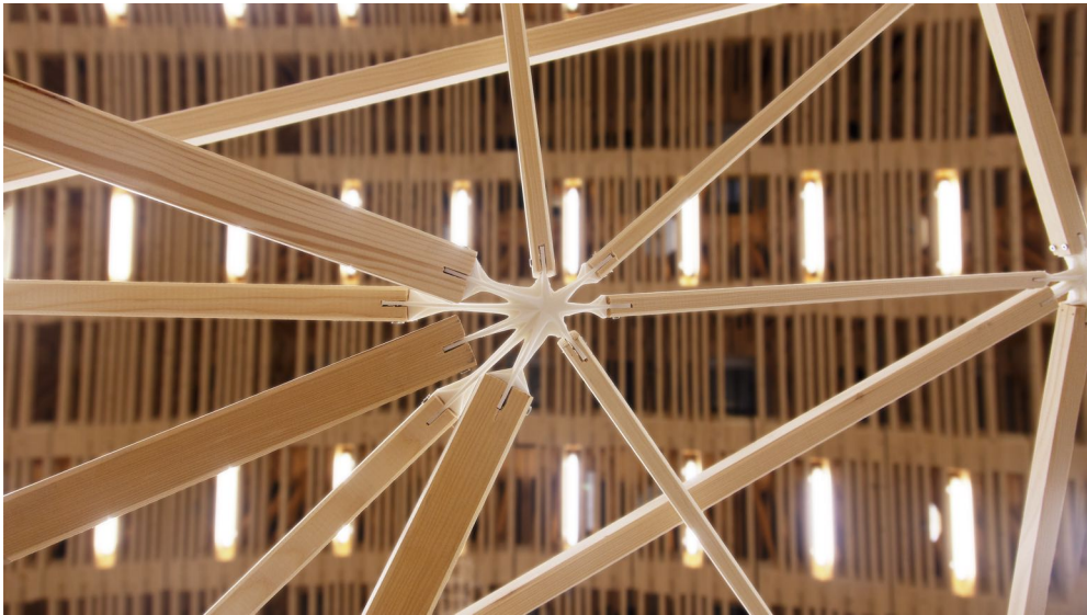
Figure 21: FDM 3D printed joint, made from PLA thermoplastic material. The node connects three members of 1st, two of 2nd, and four of 3rd hierarchy.
